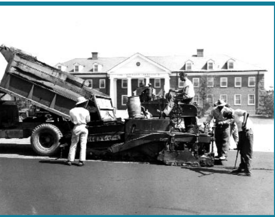
1950's Barber-Greene Paver. Former Asphalt Institute Headquarters, College Park, Maryland, is in the background.
