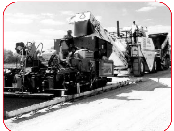
This is a Roadtec SB-2500 materials transfer vehicle placing the mix into a Blaw-Knox paver on U.S. 68 near Bowling Green, Kentucky, in 1998.
