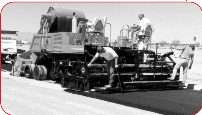
This Barber-Greene MTP-1260 is equipped with a windrow pick-up attachment. The hot mix is dumped from bottom-dumping trucks, then picked up and placed into the paver. This is a 1989 job.
