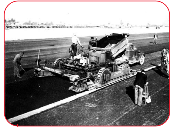
A Jaeger spreader on an airport runway surfacing project using a side-form control in the 1940's.
